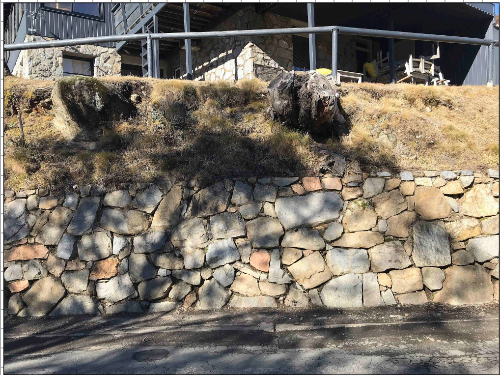
Plate 1: front elevation of rock wall immediately downslope of proposed new post for deck extension. Erosion of soil from behind the wall evident.
